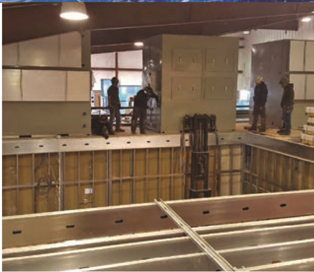
MSP's dehumidification technology is also used in archives, clean rooms and indoor swimming pools. Courtesy Photo
